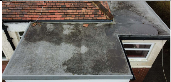
Flat roof – there does not look to be enough fall on the flat roof as there are areas of ponding.
