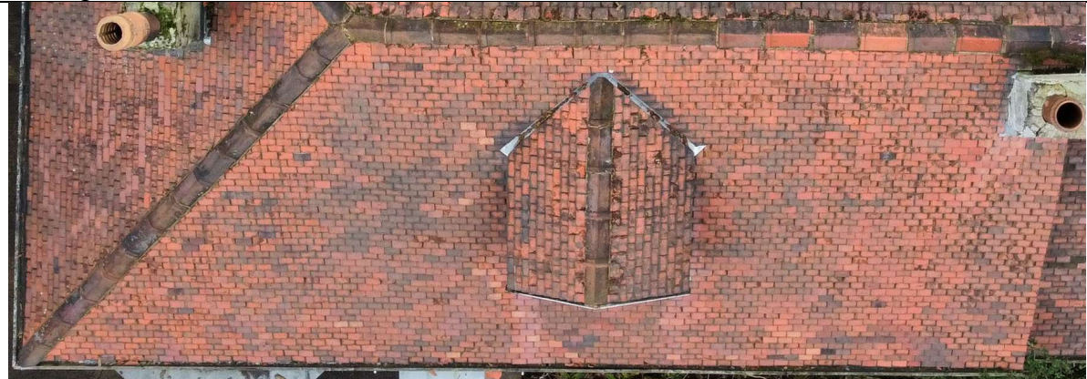
Hip and ridge pointing – this is coming away in places along the length of the hip and ridge. The defective pointing needs to be removed and replaced, preferably with a hot lime-based mix to maintain flexibility.
