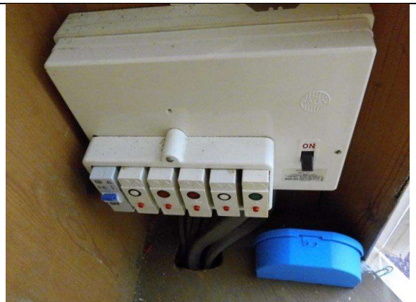
Distribution board – second-floor landing cupboard.
