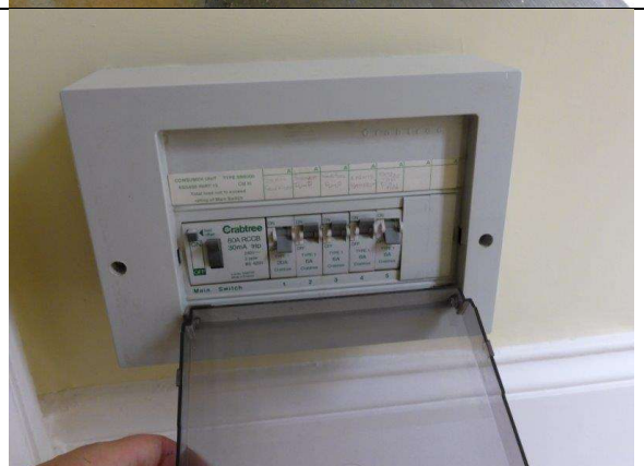
Distribution board outside bedroom two.
