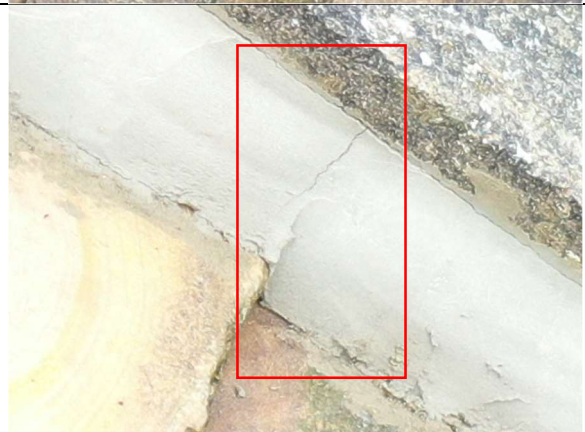
Parapet detailing – example of a hairline crack that has formed in the mortar fillet.
