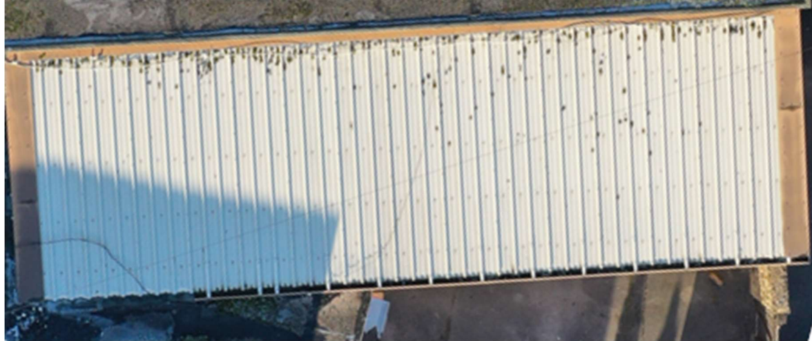
Example photos of cut edge corrosion at the foot of the roof. This should be treated in the short term to prevent further deterioration of the sheets.
