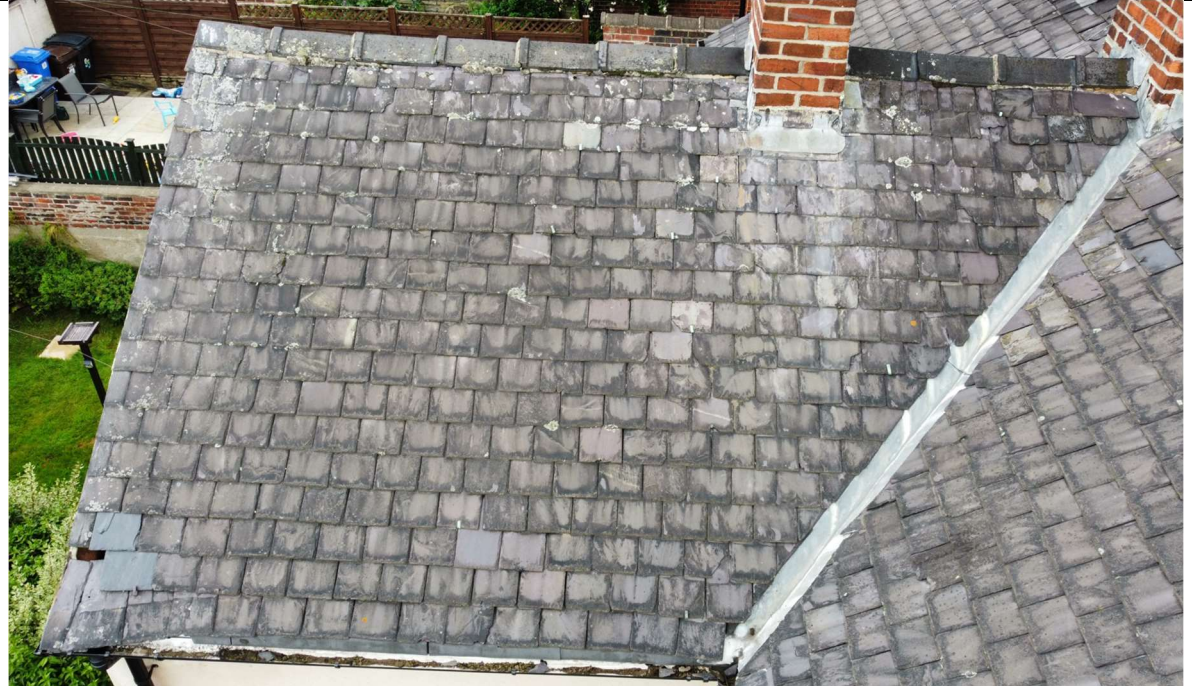
Ridge – there are sections of damaged and missing pointing. The ridge should be raked out and repointed before winter.
