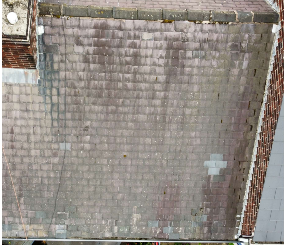
Overhead photo of the front roof pitch. Note the heavy staining to the slates.
