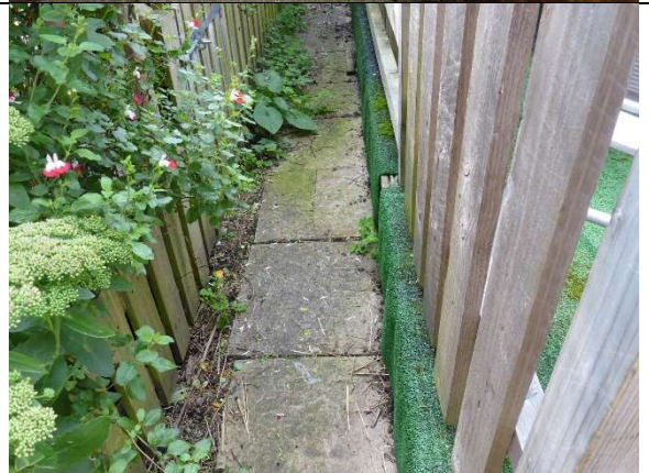
Left-hand side path – there are several damaged paving slabs along this path. These should be replaced in the short-medium term depending on if the pathway will be used.
