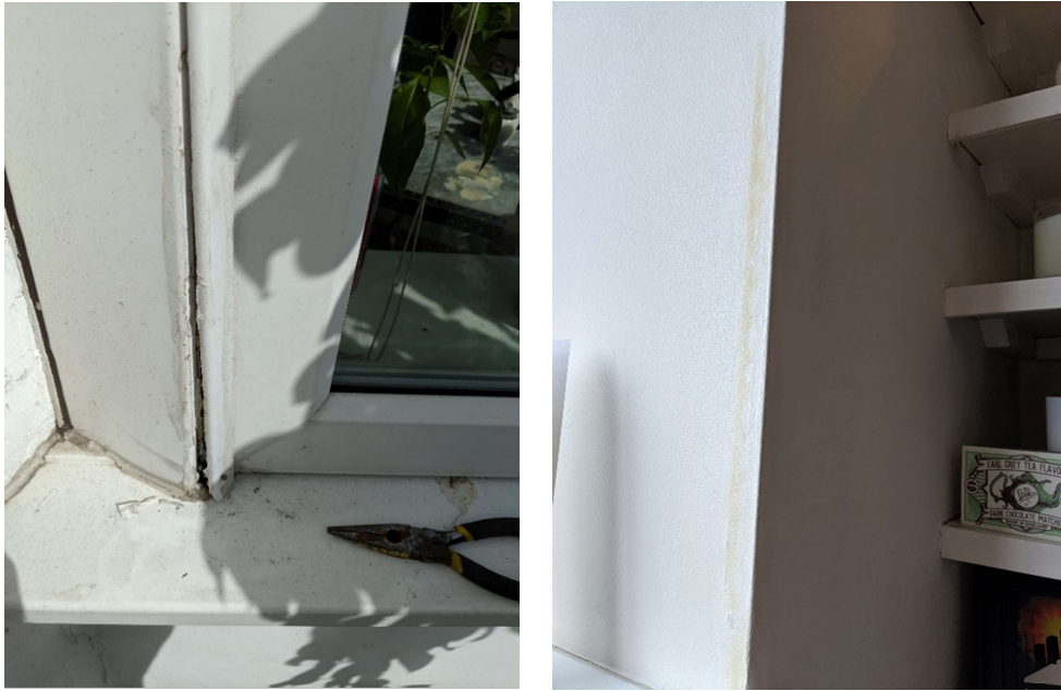
Fig. 23 – The silicone bead sealing the window trim to the frame has been removed to leave the trim loose (left) and brown staining to the finish on the inside of the bay window (right).
