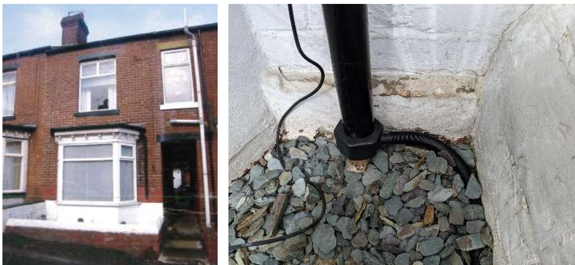
Fig. 19 – Missing bottom section of fall pipe (left) and water butt connection modification to fall pipe (right).
