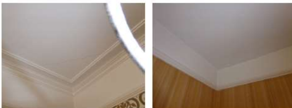
Example of cracks to ceiling
