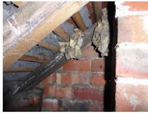
Salts and staining to timbers and repairs
