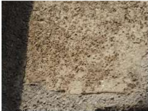
Cracks around the joints were repairs have been undertaken
