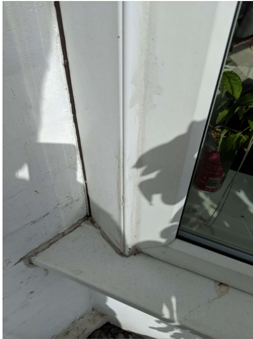
Fig. 17 – uPVC window trim.
