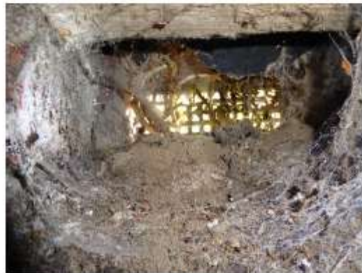
Blocked up air vent
