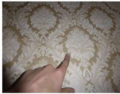
Crack going down the stairs
