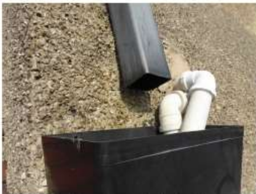
Downpipe not correctly discharging
