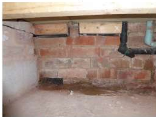
Plastic DPM visible and moisture at the base of the wall
