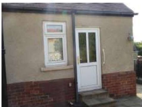
Section of rebuilding and new render which has a vertical crack
