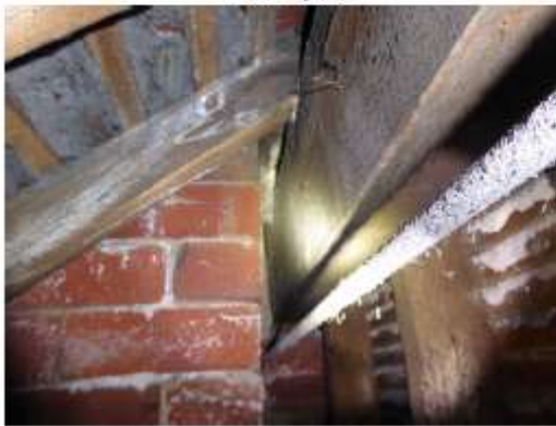
Salts around chimney breast
