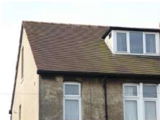
Slipped / missing tiles / dormer
