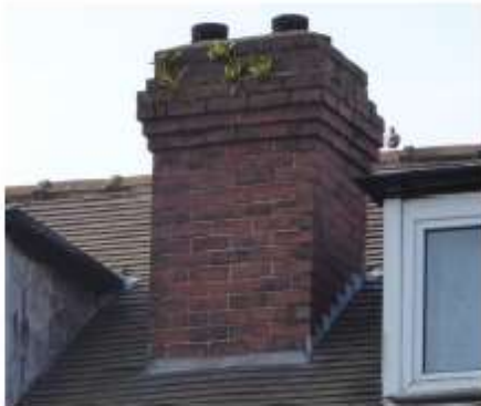
Front chimney stack – vegetation / loose pointing / dated leadwork
