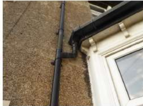
Staining to downpipe
