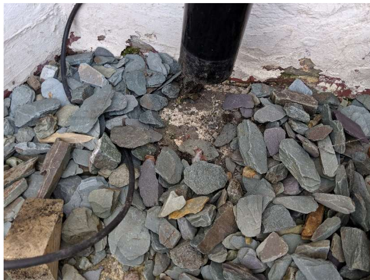
Fig. 24 – Fall pipe with water butt connector removed.
