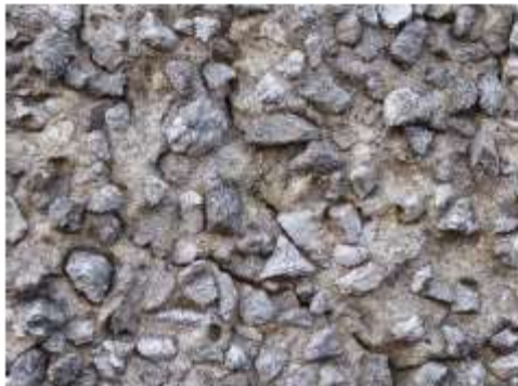
Example of cracks to render
