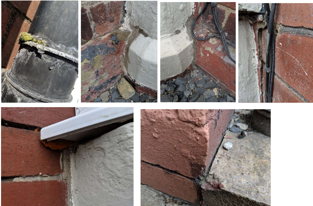
Fig. 49 – Case Study One Defects.
