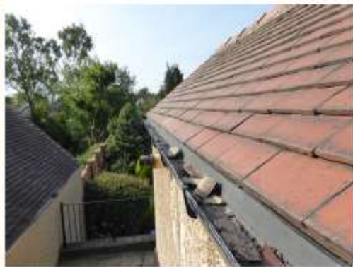
Gutter full of debris
