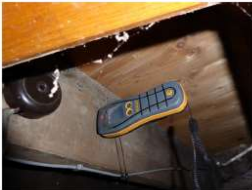
Moisture meter showing high readings
