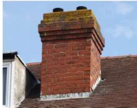
Rear chimney stack – lichen / loose pointing / dated and loose leadwork
