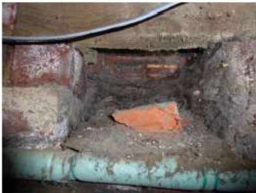
Blocked up air vent
