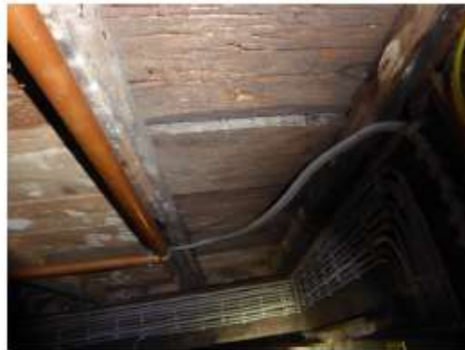
Decay to timber floor under porch
