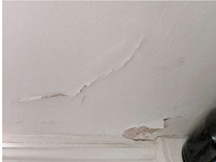
Fig. 21 – Signs of Damp on living room wall.
