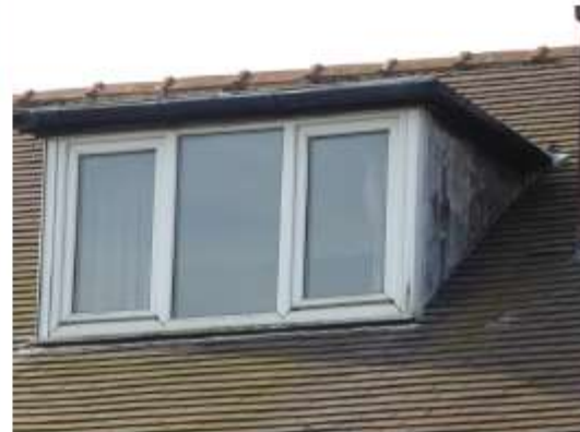
Slipped / missing tiles / dormer
