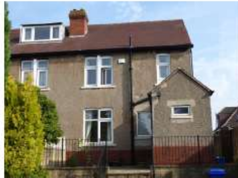
Areas of repairs and Staining
